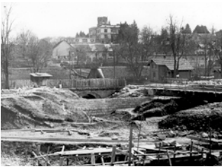
Construction of railway tunnel and rerouting of the River Sihl around 1919. Photo: Archive of Building History, City of Zurich.
